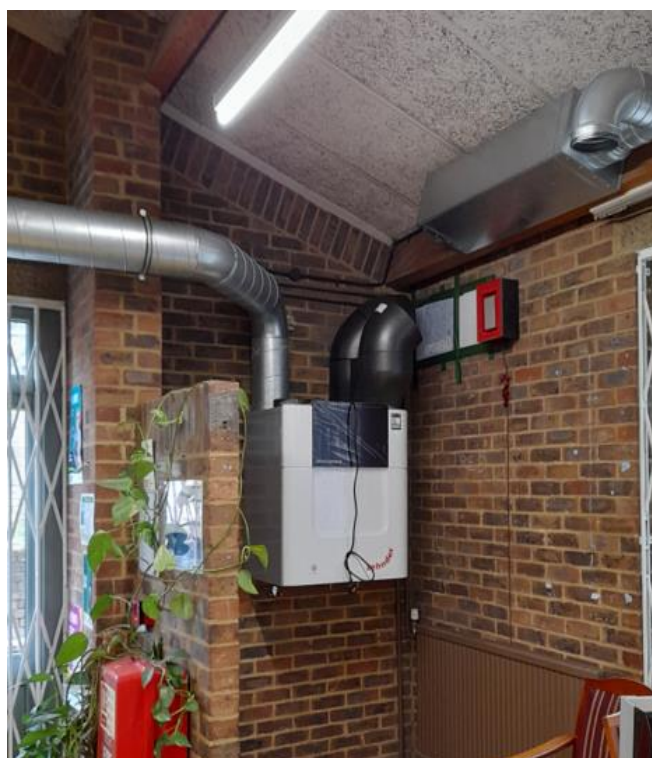
Mechanical Ventilation with Heat Recovery unit installed in one of our spaces May 2023
